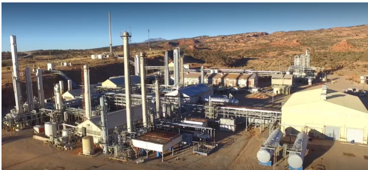
Paradox “5.5 Nines” Resources Lisbon Valley Gas Processing Plant.
