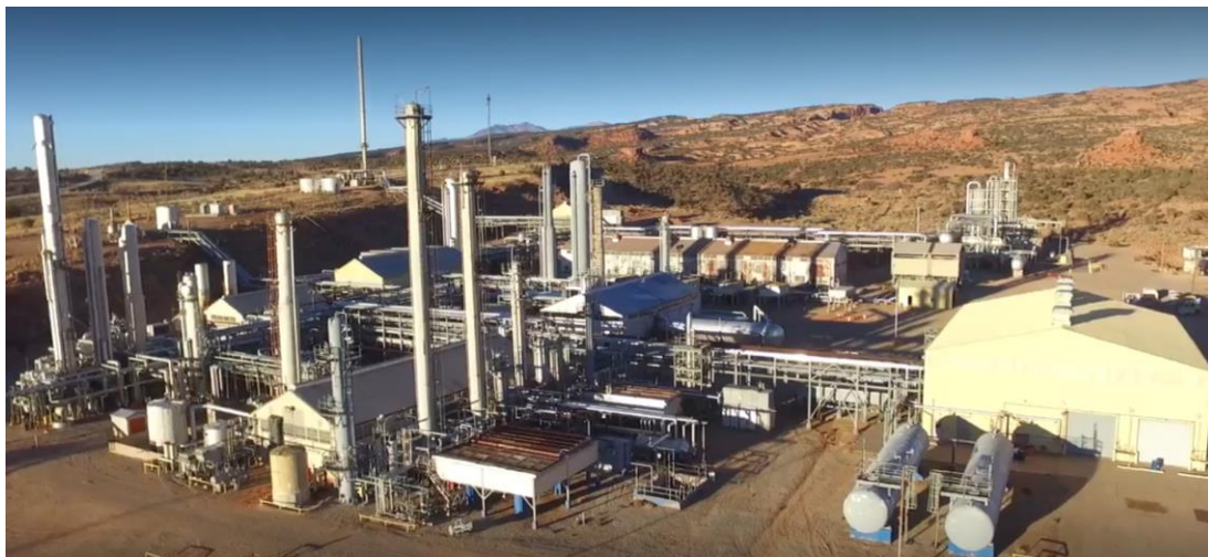
Figure 3: Paradox “5.5 Nines” Resources Lisbon Valley Gas Processing Plant.
