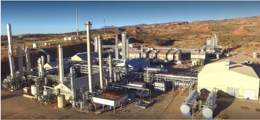
Figure 3: Paradox “5.5 Nines” Resources Lisbon Valley Gas Processing Plant.
